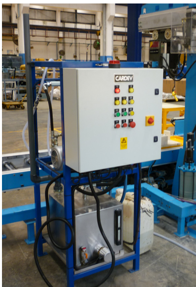
Critical Port Flushing Station
